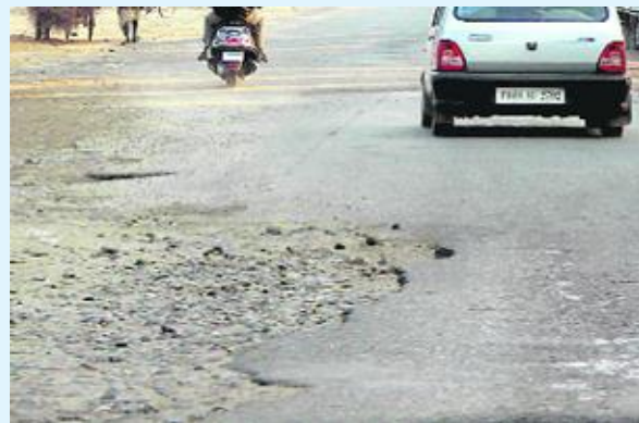
b) Rough road surface condition
