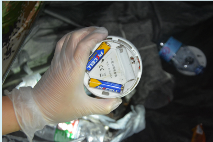
One of the batteries fell off and could not work normally. Figure 3: Carbon Monoxide Alarm Found on Site.
