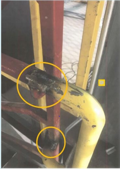
Figure 12: Photograph of Handrail with the Welded Areas Circled in Yellow.
