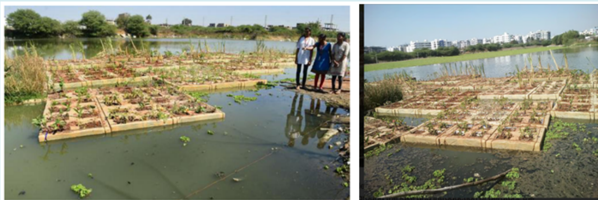
Figure 4: Installation of the floating treatment in the historic Nekkampur Lake in Hyderabad, India (Lakes of India https://lakesofindia.com ) [50].
