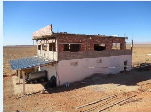
Figure 3: The farmer is constructing a building for the irrigation machinery that includes adding nutrients to the water in carefully calculated doses.
