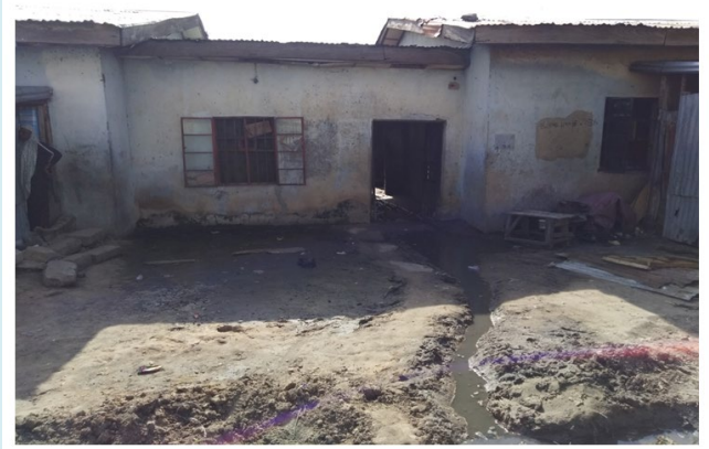
Figure 7: Entrance to an overcrowded dilapidated apartment at Old Maiduguri district.
